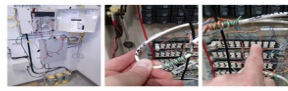
--- Troubleshooted and fixed PVT'S phone line connections and repaired them in this site (DNAMC - 2012) in Roscoe. --- Found the repaired PVT'S lines for that site and did in quality and
